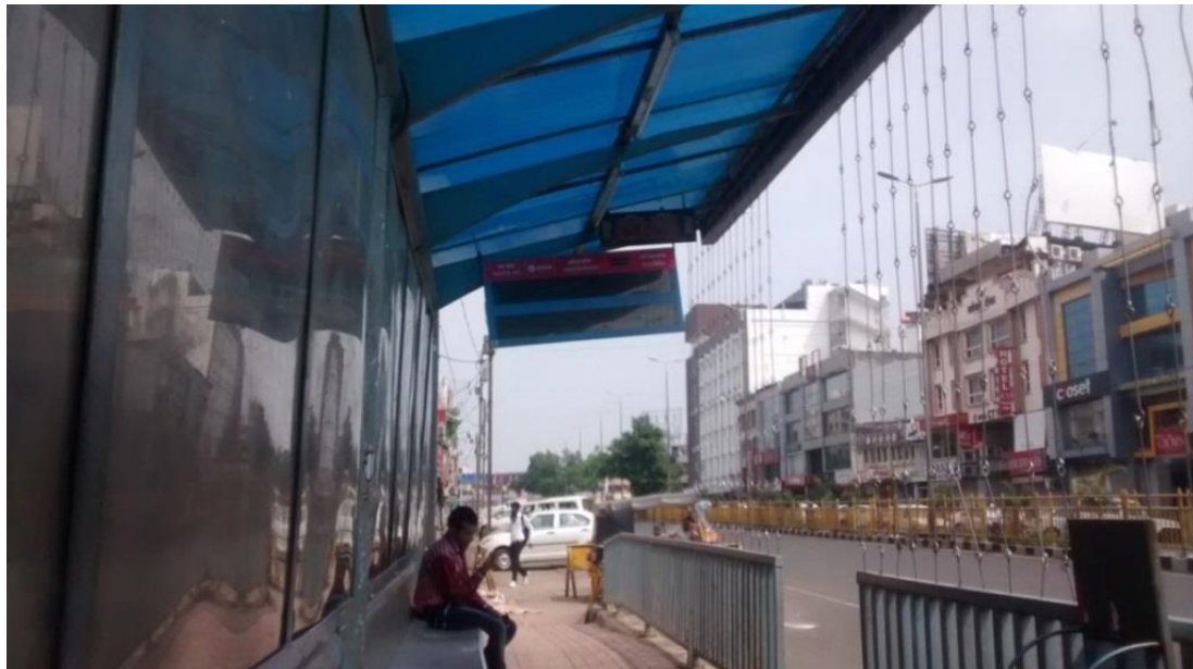
Figure 5.20: Non-functional display boards, New Market.
