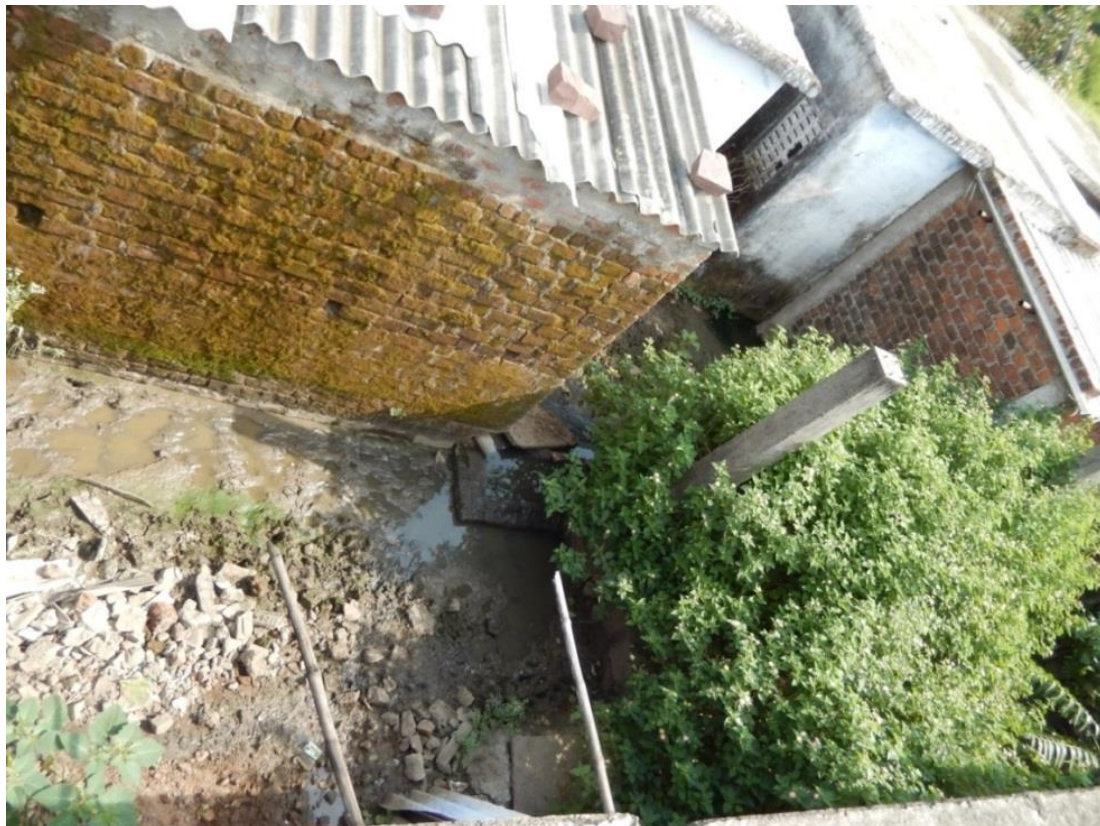
Figure 5.11: Overflowing septic tanks, Hinotiya Alam.
